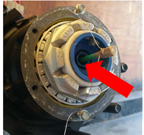
Soap check along rotating shaft back into spindle plug for leaks
